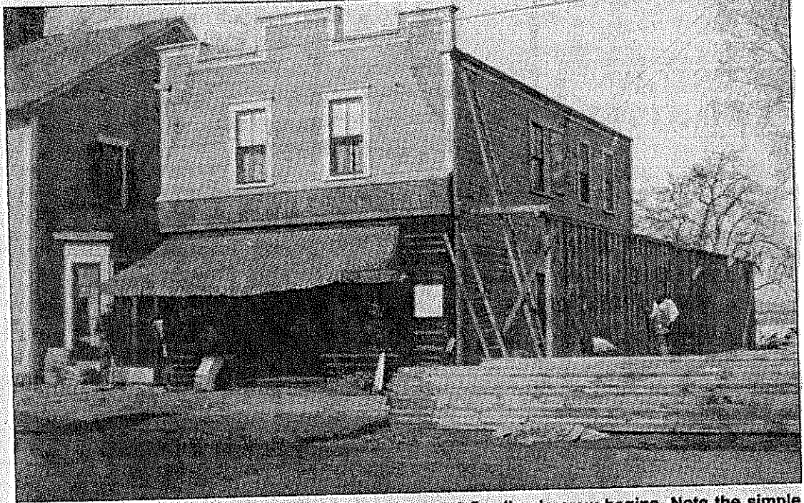
With both small stores gone, construction by Howard Gardiner's crew begins. Note the simple 20th-century windows in the second floor.
